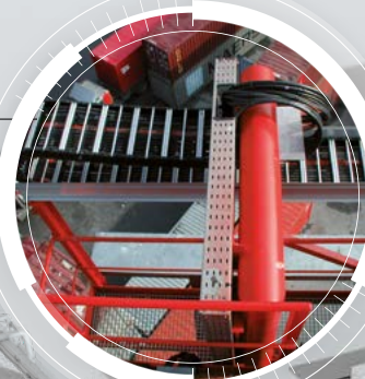
Rail Mounted Gantry [RMG]
