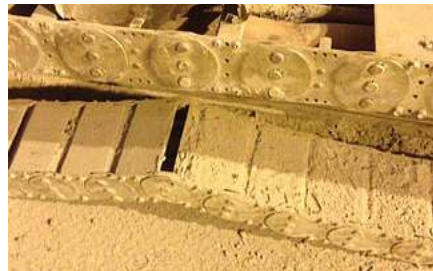
Negative example: Cover system with high dust accumulation
